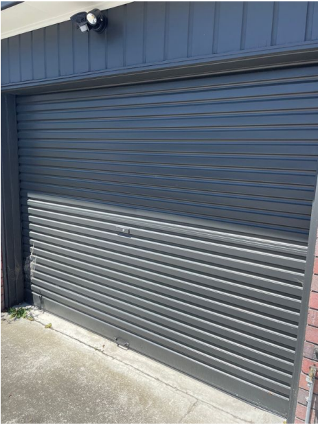
Garage Door: Material & Type Metal, Automatic, Roll-Up
